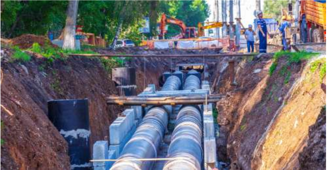
Repair work in the city to replace water pipes in the city of Samara, Russia © Shutterstock
